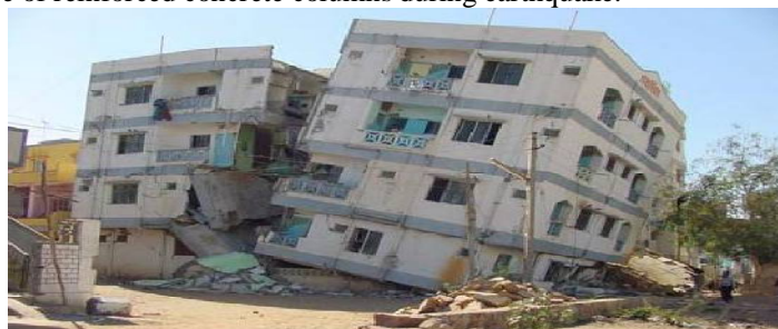
Fig.1 Collapse of reinforced concrete columns (and building) during 2001 Bhuj (India) earthquake
